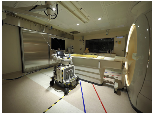
Fig. 3. Tethering of mobile MR imaging unsafe equipment in Zone 4 in interventional MR imaging suite. Note the fixed-length cable tether system that limits movement of the ultrasound system to the (caution) yellow and black striped floor markings at a distance from the magnet. The yellow and black marking matches that on the ultrasound system chassis. The red line marks 300 Gauss; the blue line marks 100 Gauss. (Courtesy of Dr. K. Gorny, Mayo Clinic, Rochester, MN.)
